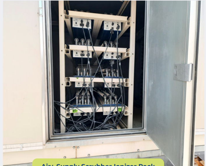
Air+ Supply Scrubber Ionizer Rack
