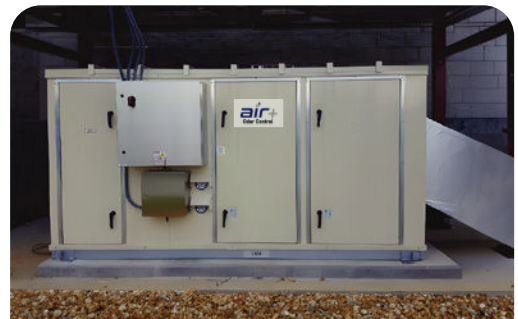
Supply Scrubber Serving Headworks Building
